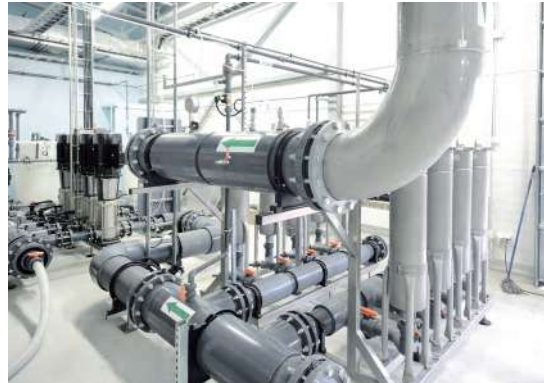
Municipal water supply
