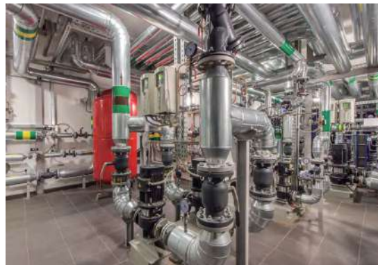
Municipal heating system
